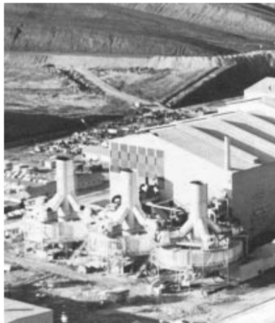
Fig. 8.34 Induced draft rotary or circular sinter coolers, shown in process of construction.
