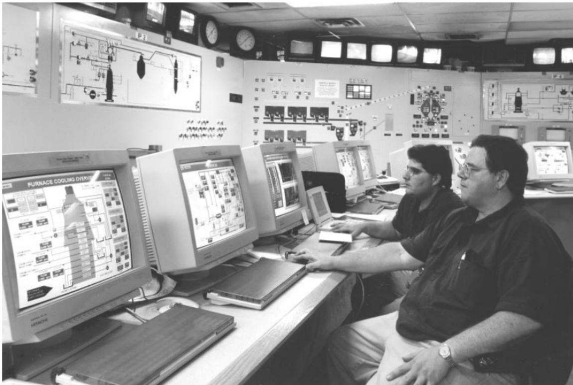
Fig. 10.4 Real time status of the stoves is reviewed in the control room. (Courtesy of Kvaerner Metals.)
